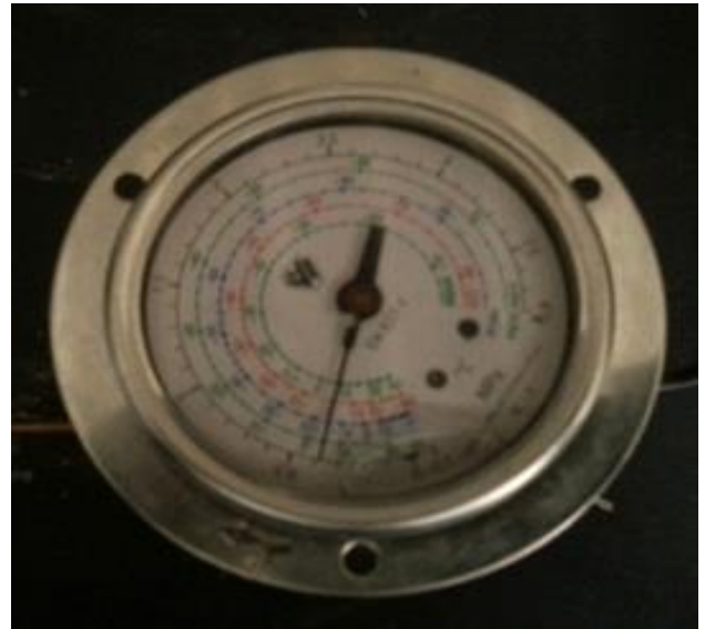
Fig 7: Shows the Pressure & Temperature Gauge
