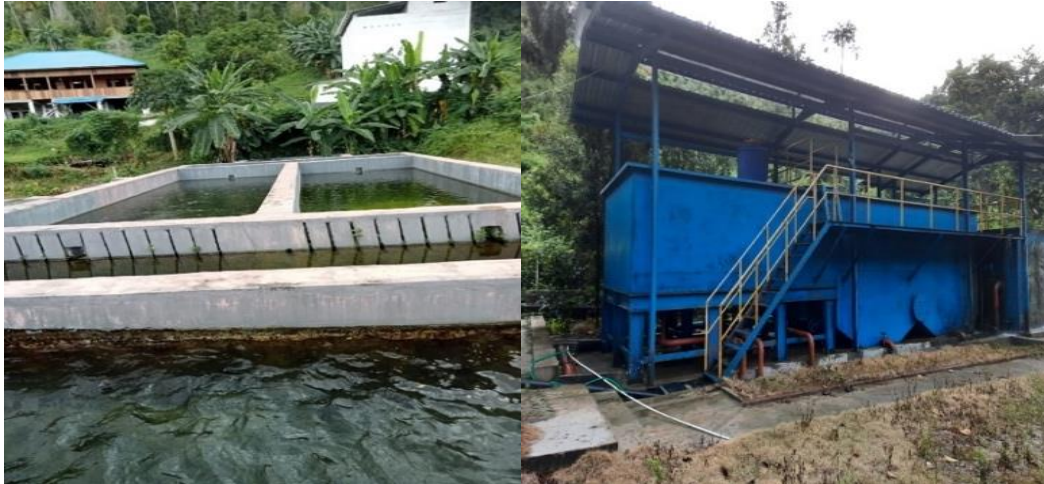
Fig. 2: Water Treatment Plant and Saluba Storage Tank
