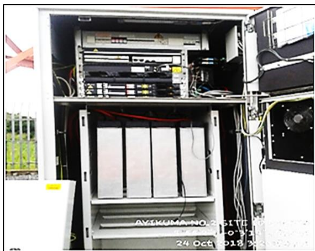
Fig 3 MPPT, Converter and Bank of Batteries
