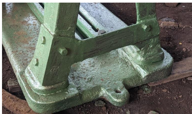
Fig 14 Broken Leg after Corrective Maintenance
