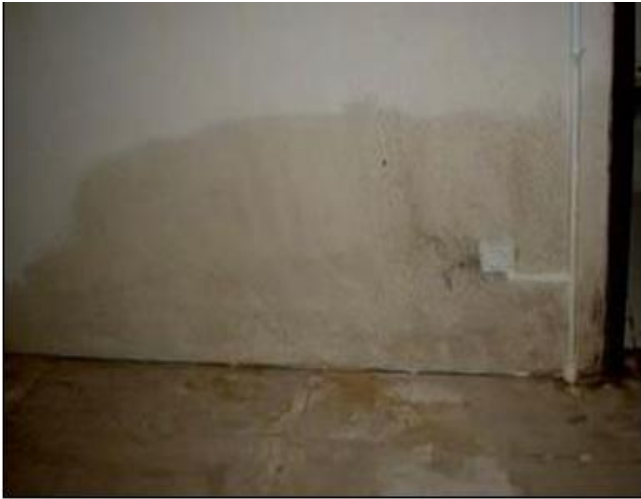
Fig 2 Rising Dampness Problem
