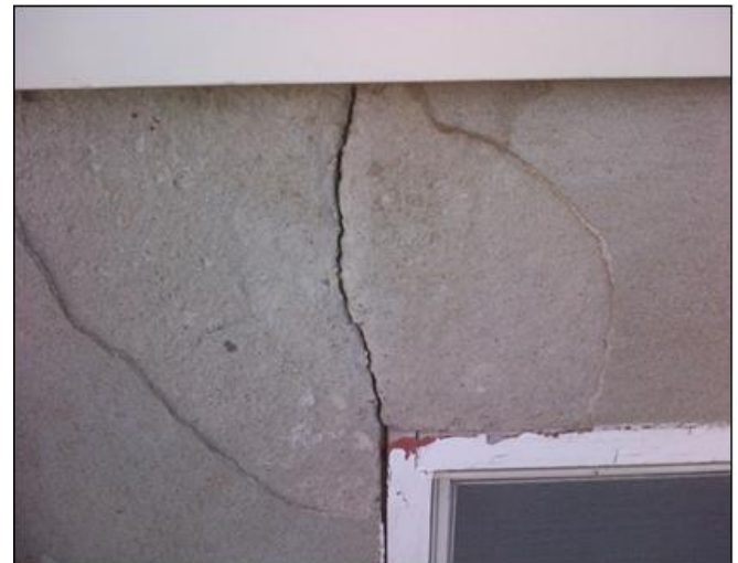
Fig 1 Crack between bay Windows Corners
