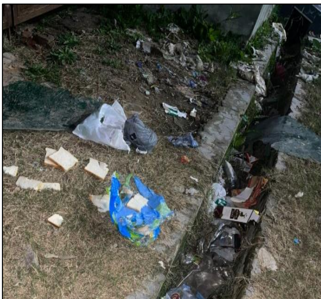
Fig 2: Waste Clogging the Drainage System Leading to Contamination of Water in Nigeria (Source: Field Survey, 2024).
