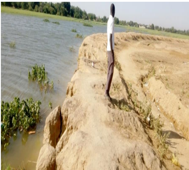
Picture 6 Dike Protecting the District from River Water Source: Gassina P., September 2020
