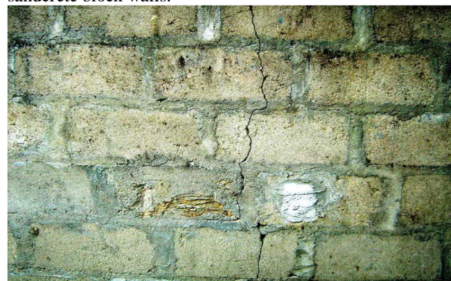
Fig 1 A typical sandcrete wall failure in Ogbomosho, Nigeria
