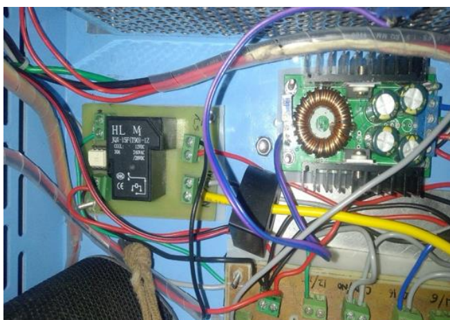
Fig 10 Boost Converter and DC Relay
