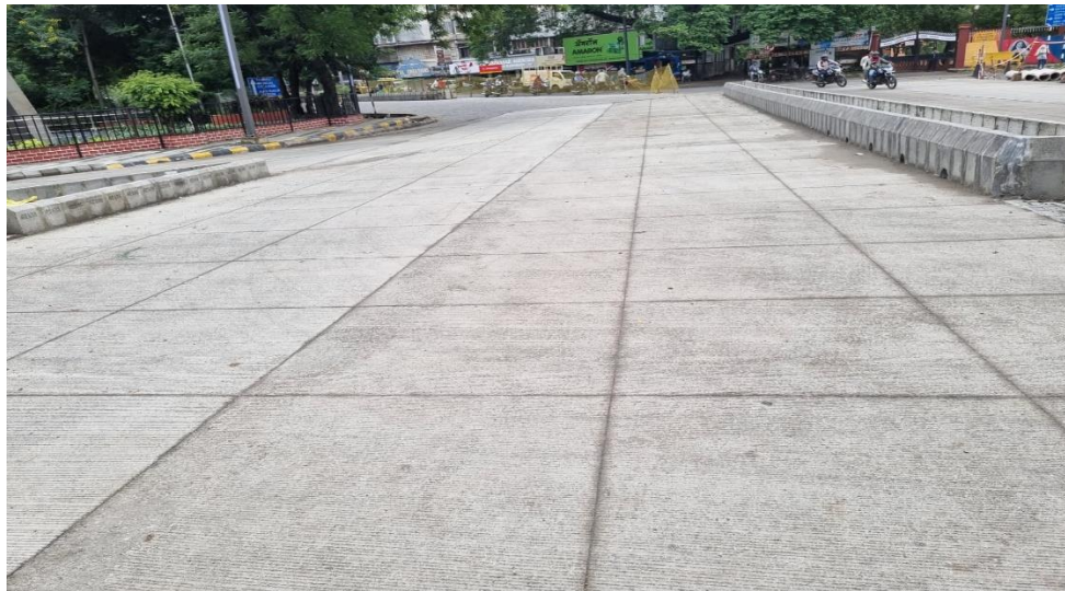
Fig 3 Thin White Topping Work Done on The Side Road at Ajni Square on Nagpur -Wardha Road
