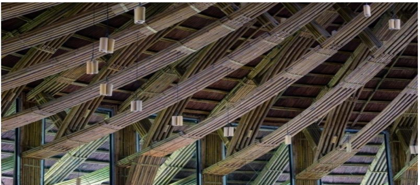
Plate 3 Bamboo as Roofing Materials (Trusses Detail) in a Restaurant: Serena Resort Bamboo Restaurant, HoaBinh, Vietnam. Source: BambuBuild (2019) http://www.bamubuild.com/en
