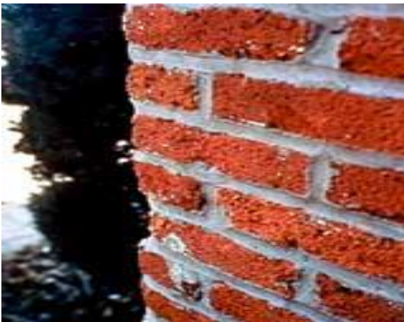
Fig. 6: Permanent Damage Done On Masonry Façade Due To Abrasive Cleaning
