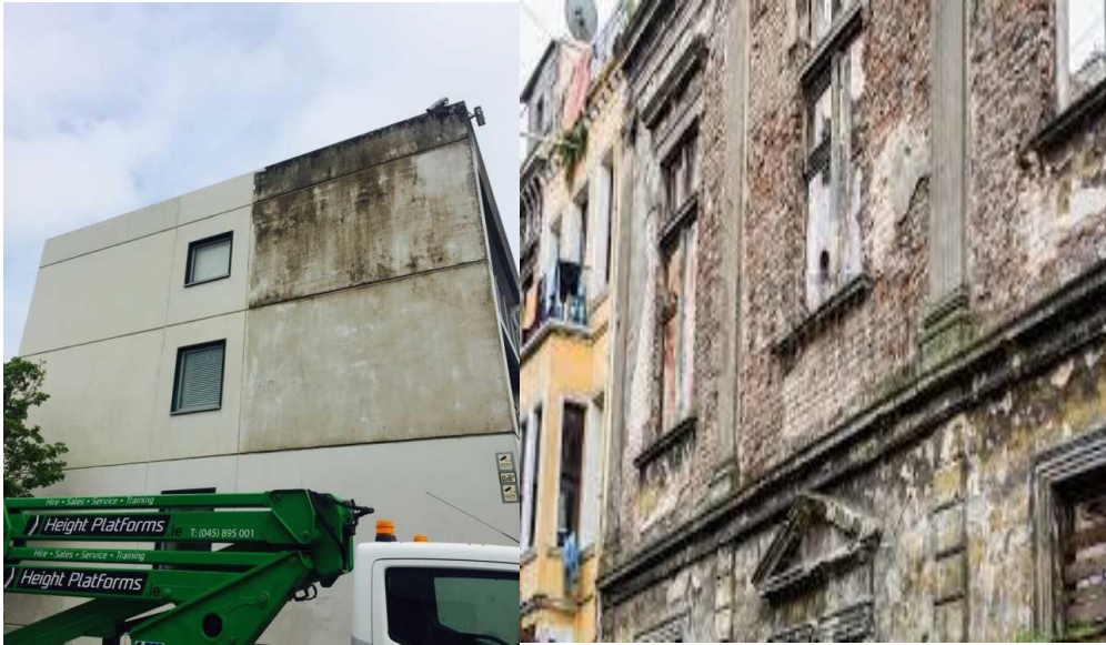
Fig. 7: Neglected Facades Showing Signs Of Rot And Degradation (source: pmac.ie, 2022)
