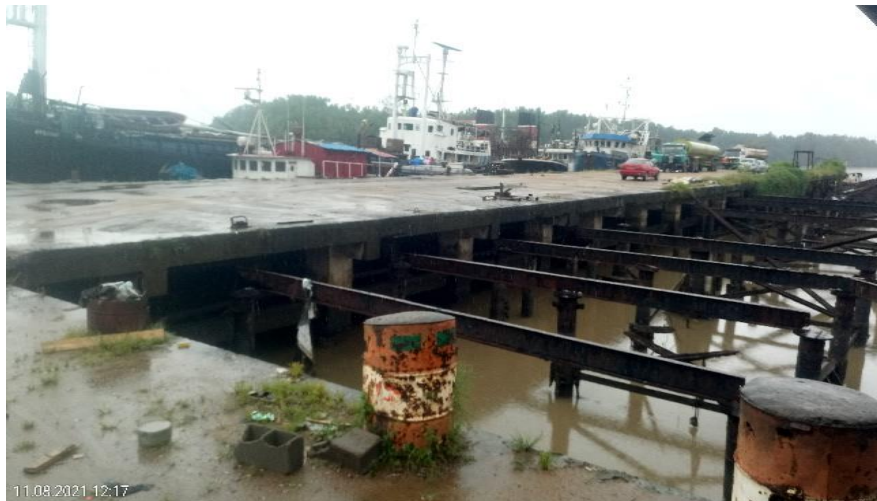
Photo 2: A dilapidated jetty at the Tiko seaport
