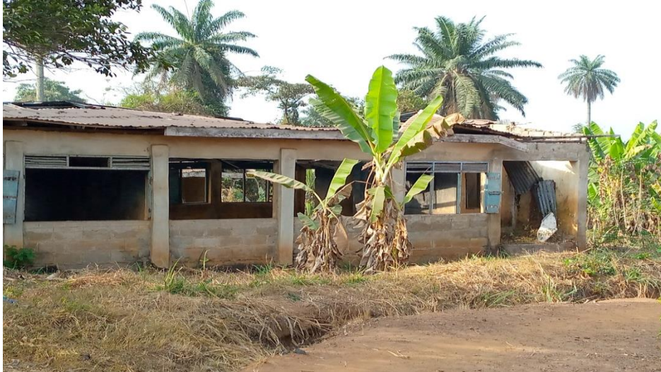
Plate 1: The block of classroom damaged by storm and abandoned due to incessant destructions year in and out in Oranmiyan Memorial Grammar School, Ile-Ife.
