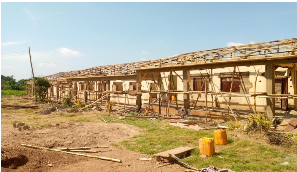
Plate 3: Building under rehabilitation after being damaged by storm at Oluorogbo High School, Ile-Ife
