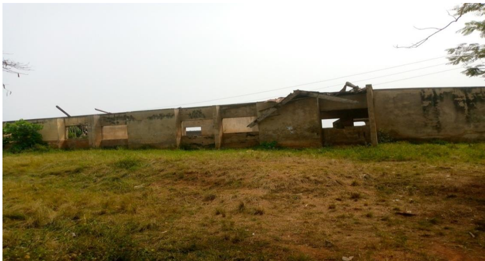
Plate 2: The block of classroom outrightly carted away by storm in Oluorogbo High School, Ile-Ife
