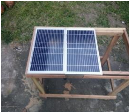
Fig 1:- Physical Form of Solar Module mounted on frame
