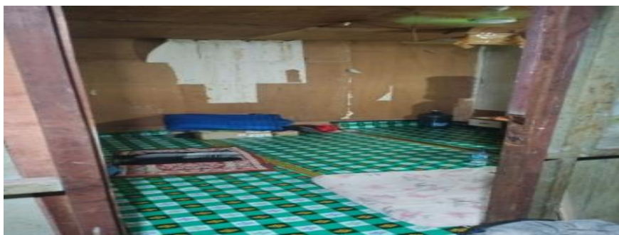
Fig. 6: Wrong condition 1 bedroom
