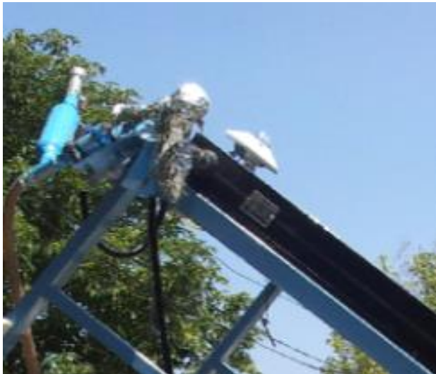
Fig 2. Position of the pyranometer
